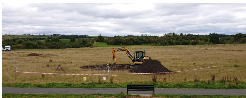
Top: newly created pond with dipping platform at Bannockburn High School, Stirling Bottom: creating a new pond at Hallglen Policy Bing, Falkirk
